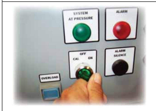
Figure E-7 Power Switch to CAL
